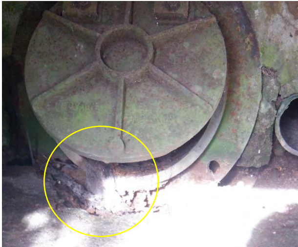
Plate 4-20: Outfall with control valve. This was not active on day of survey but rags are visible in the pipe (yellow circle) indicating it discharges foul water.
