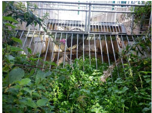
Plate 4-15: Glasheen just before it enters the culvert diverting it under the carpark at Dunnes and the N40 road.
