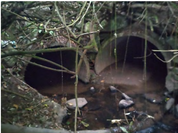
Plate 4-16: Pipe culvert on the left is the outfall of the Glasheen after it is diverted under the South Link Rd. Pipe on the right is an unknown piped stream.
