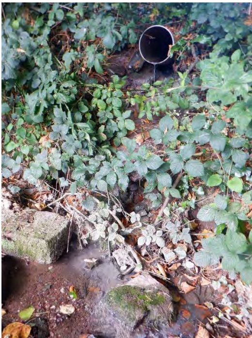
Plate 4-18: Outfall pipe discharging grey water on the day of survey. Grey water in the stream is visible in the bottom half of the photograph
