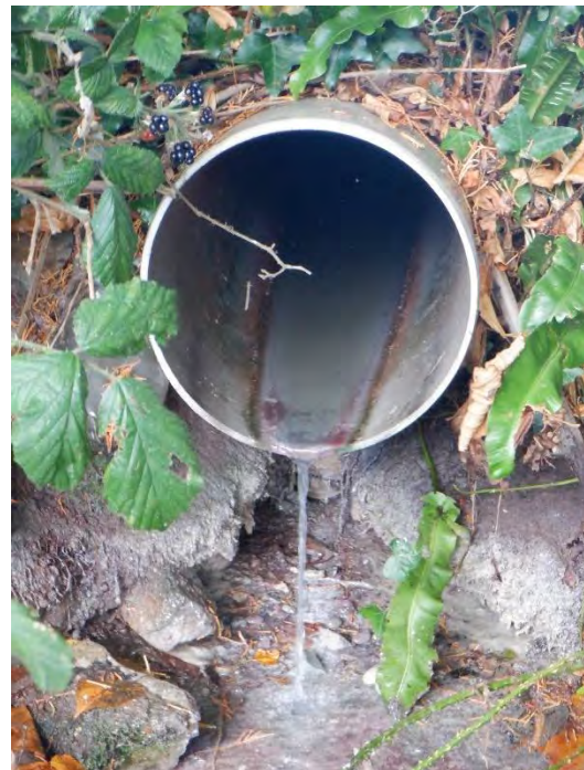
Plate 4-19: Close up of the pipe in previous image with sewage fungus visible around the outfall.
