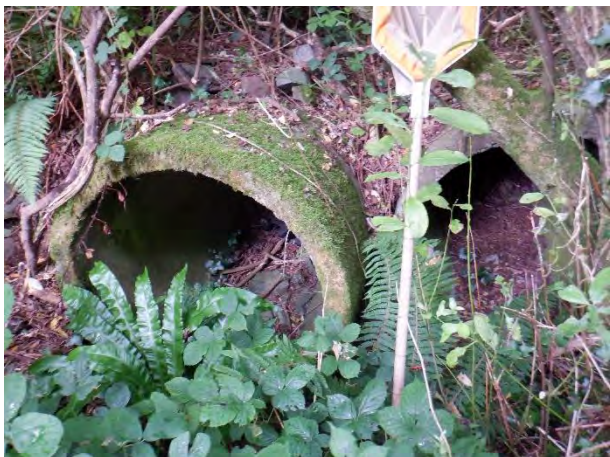
Plate 1-1: Old pipes which brought water from the Two Pot to the Glasheen.
