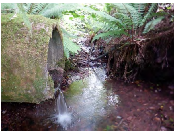
Plate 4-5: Outfall of a small stream to the Glasheen which is piped under the cemetery. See Figure 1-2 for historic mapping of this channel.
