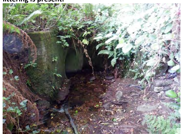
Plate 4-6: The Glasheen just before it is diverted under the Bandon Rd through a pipe culvert.
